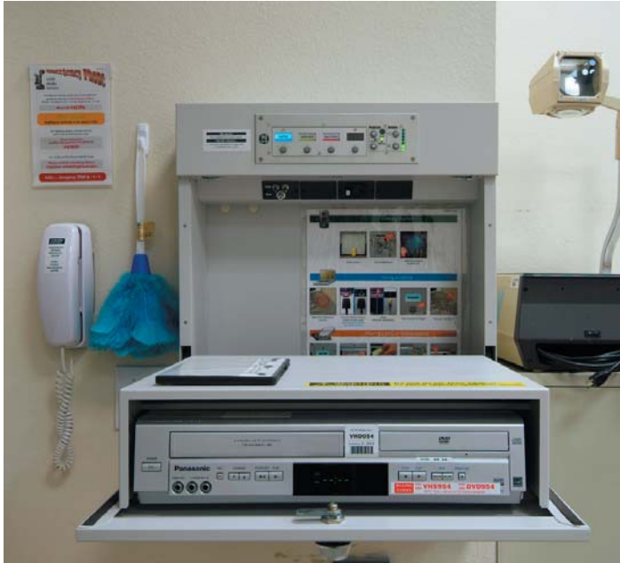
Typical classroom installation. Setup in each location is identical, making it easy for teachers to use the AV equipment in each room.
