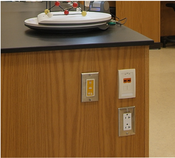
A closeup of an AV cabinet. The Pixie controller on the left is the same size as the power outlet, and eliminates the need for remotes for the projector and audio.
